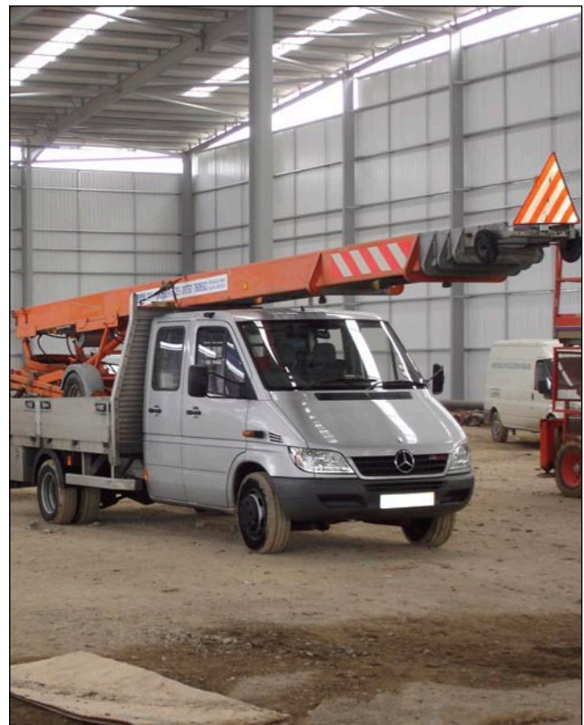
Figure 40(a) Mechanical handling of large roof sheets (Images courtesy of Advisory Committee on Roofsafety), see also Figures 5(a) and 5(b)
