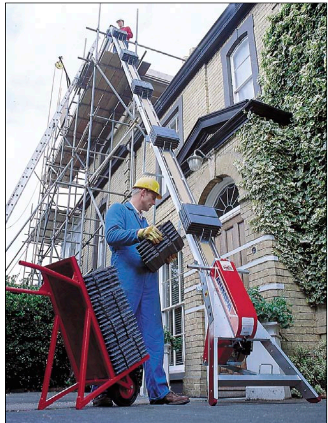
Figure 5(b) Domestic hoist
