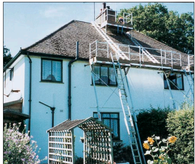
Figure 28 Proprietary system for access to roof and chimney
