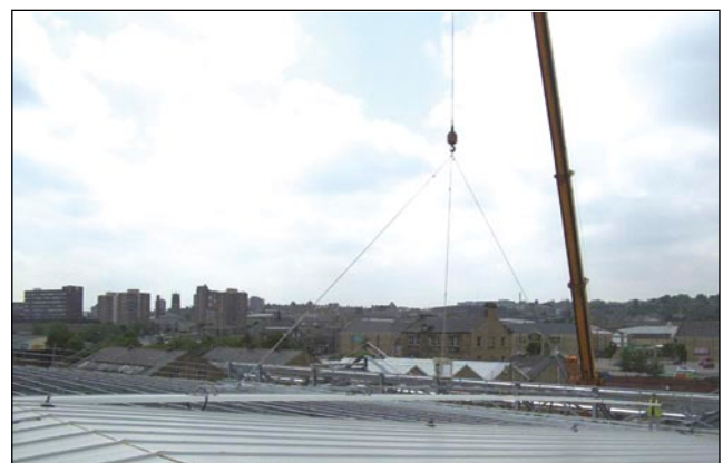
Figure 41 24 m long roof panels being mechanically lifted from ground level and installed on roof (a) (b) (c)
