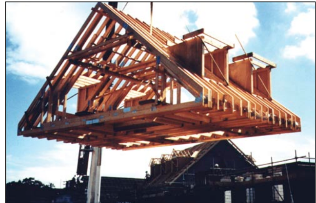
Figure 22 Craning a pre-assembled roof into position greatly reduces the need for work at height (Image courtesy of the Trussed Rafter Association)
